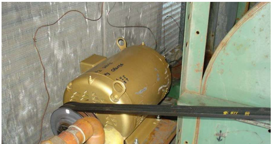
HRU-4 Supply Fan Motor, Heating Coil, and Low Limit Coil Capillary
