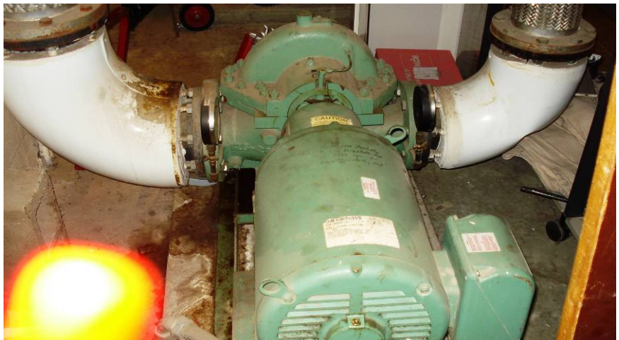
Heating Hot Water Pump
