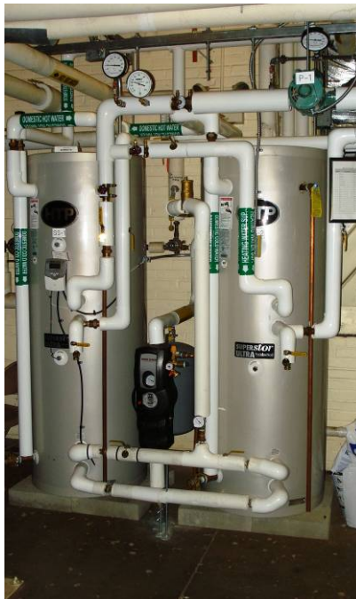
Solar Domestic Hot Water System Tanks and Gas-Fired Instantaneous Hot Water Heaters
