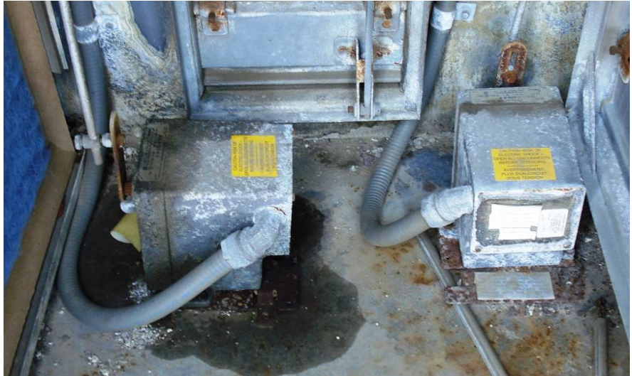
HRU-5 Intake and Bypass Damper Actuators
