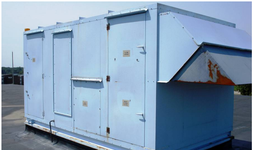
HRU-4 with Additional Intake Hood Section (right side of photo)
