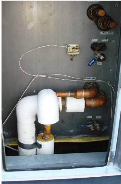
AHU-1 Coil Connections and Cardboard Covering Portion of Coil
