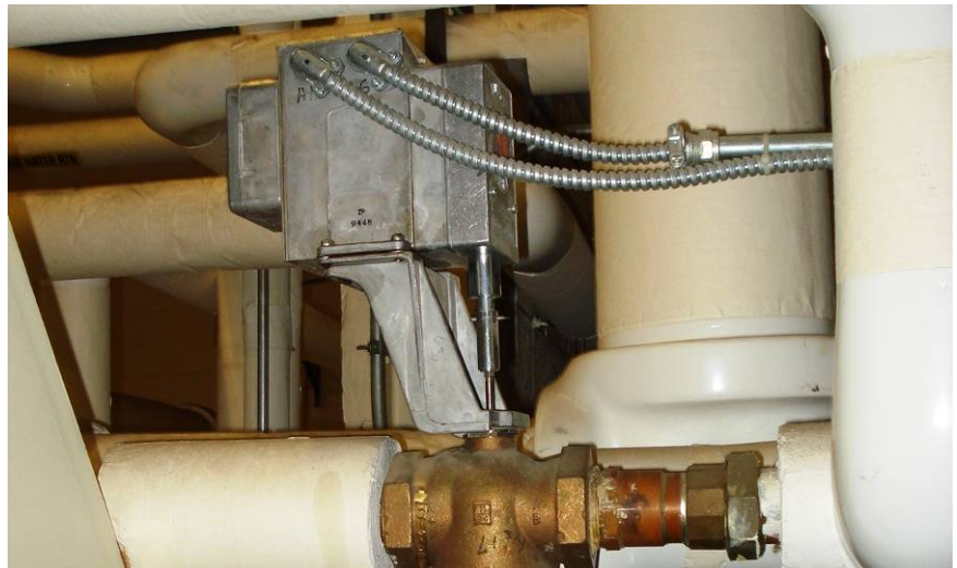
View of AHU-6 Heating Coil Valve
