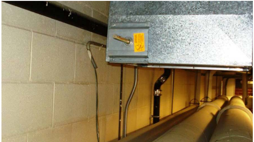
Intake Damper Associated with Exhaust Fan EF-17
