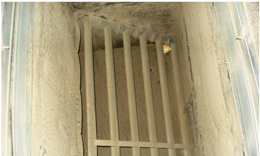
HRU-4 Dirty Return Air Plenum Duct Connection
