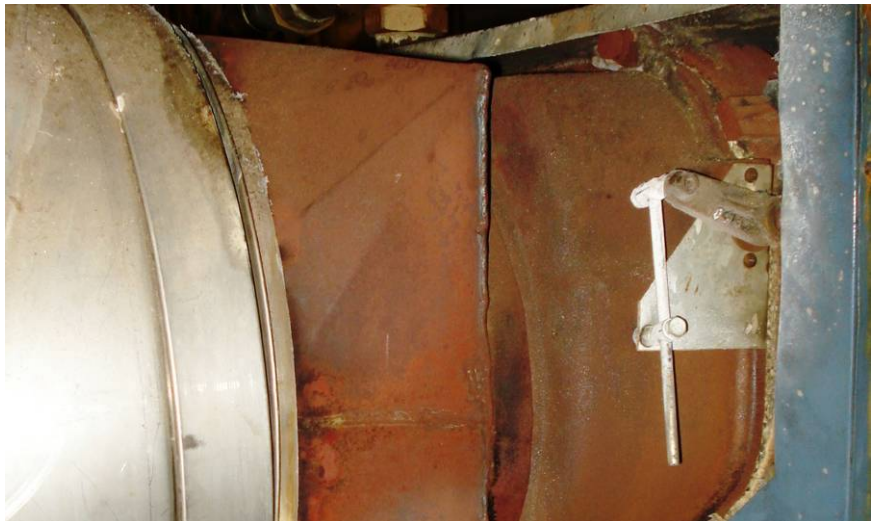
Breeching Damper at Back of Boiler 1 Was Loose
