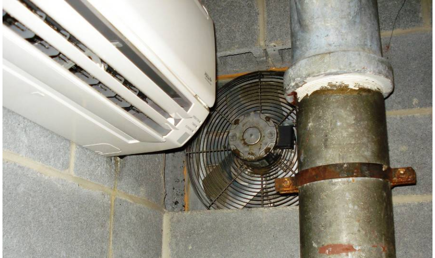
View of Exhaust Fan and Split AC Unit in Server Room E170
