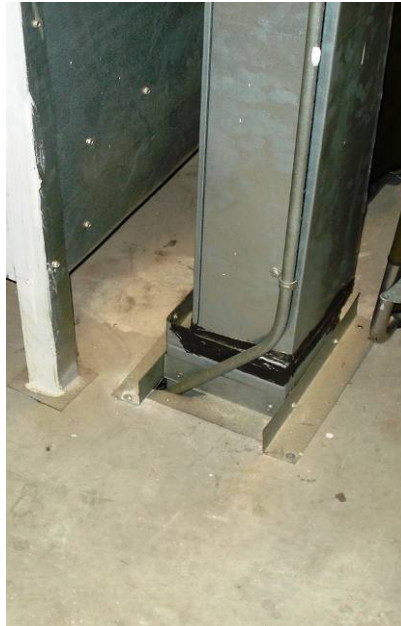
EF-7 Duct Penetrations Through Mezzanine Floor
